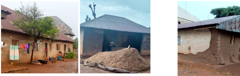
Plate 1, 2&3: State of Poor Housing Conditions in the Study Area Source: Researchers' Field Survey, 2022
